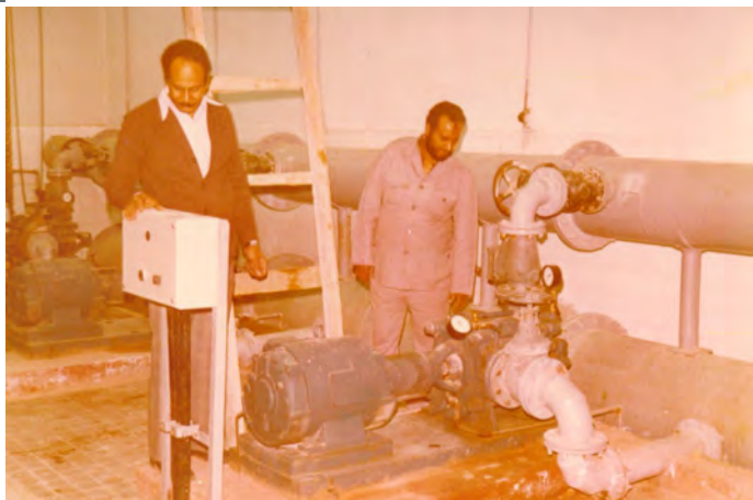
Water Pump Stations Supplied, Installed and Commissioned.
