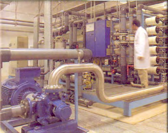
Water Treatment System Implemented by Kimans Inc.
