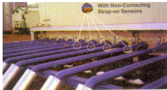
Oil Production Flow Monitoring System
